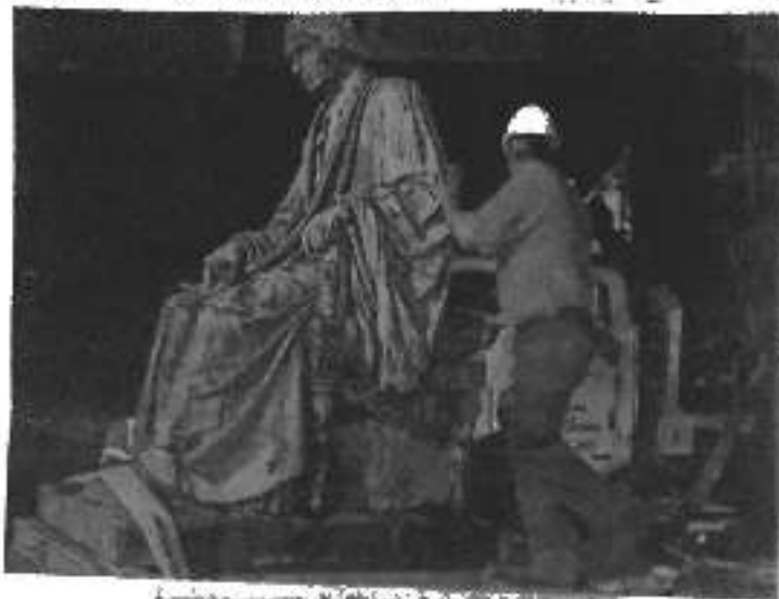
A monument dedicated to Chief Justice Roger B. Taney was removed from outside the Maryland State House.
